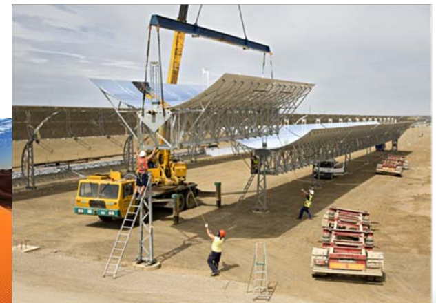
Ouarzazate CSP plant (Morocco)
