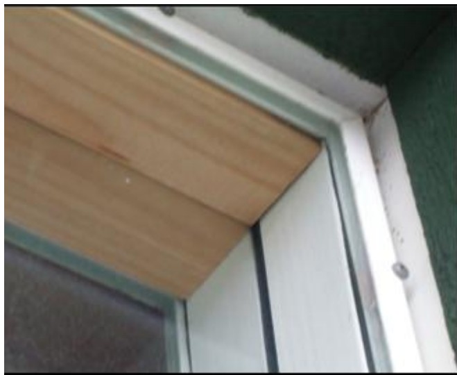
Fig. 5. A buffer of wood is placed in the top of each cavity to avoid internal condensation
