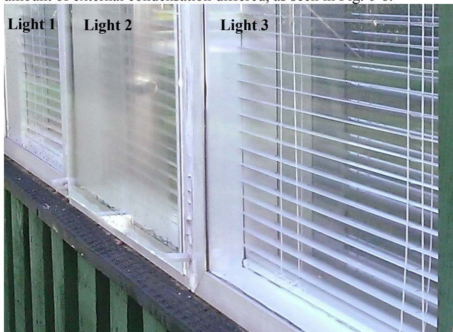
Fig. 6-8 Appearance of external condensation in the non-sealed test-window – seen from outside
