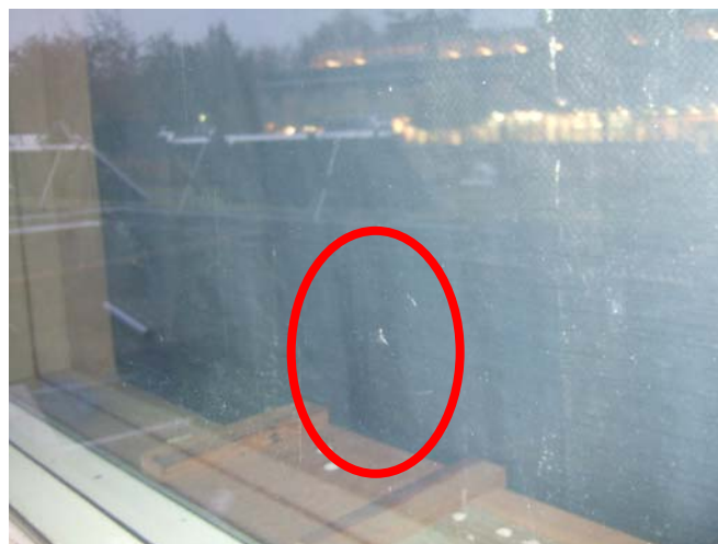
Fig. 8. Showing the “smokescreen” of adhered dust between the glazing surfaces before cleaning. The circle indicates a spot on the window where it is possible to see the striped pattern of dust on the pane. The stripes are not typical of condensation.
