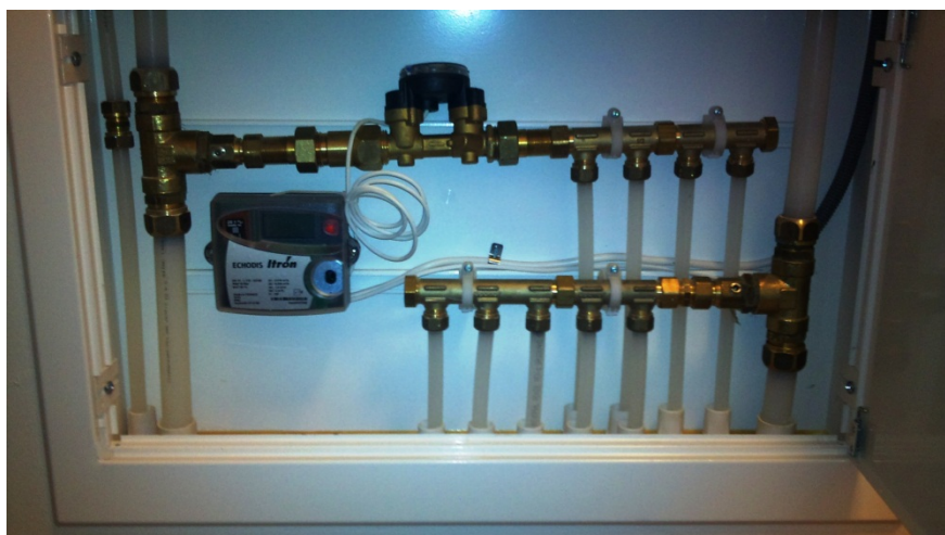
Figure 8. Installed equipment to facilitate individual metering of DHW use in each apartment. Photo: The Author.
