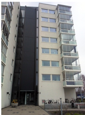
Figure 8. Solar air installation mounted above the entrance of building. Photo: The Author.
