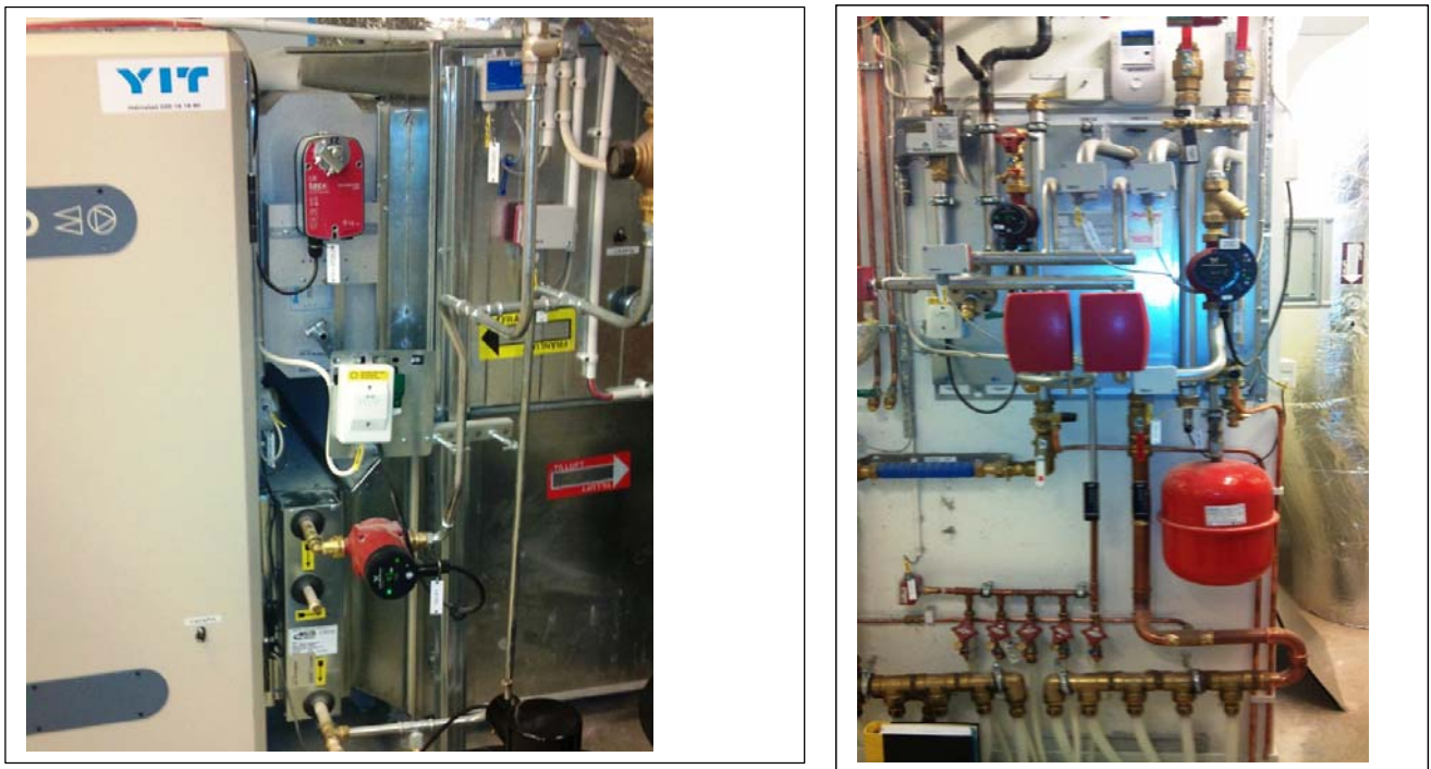
Figure 7. Close up of district heat supply heat exchanger in central air ventilation system (left), and district heat supply heat exchanger for DHW (right). Photos: The Author.
