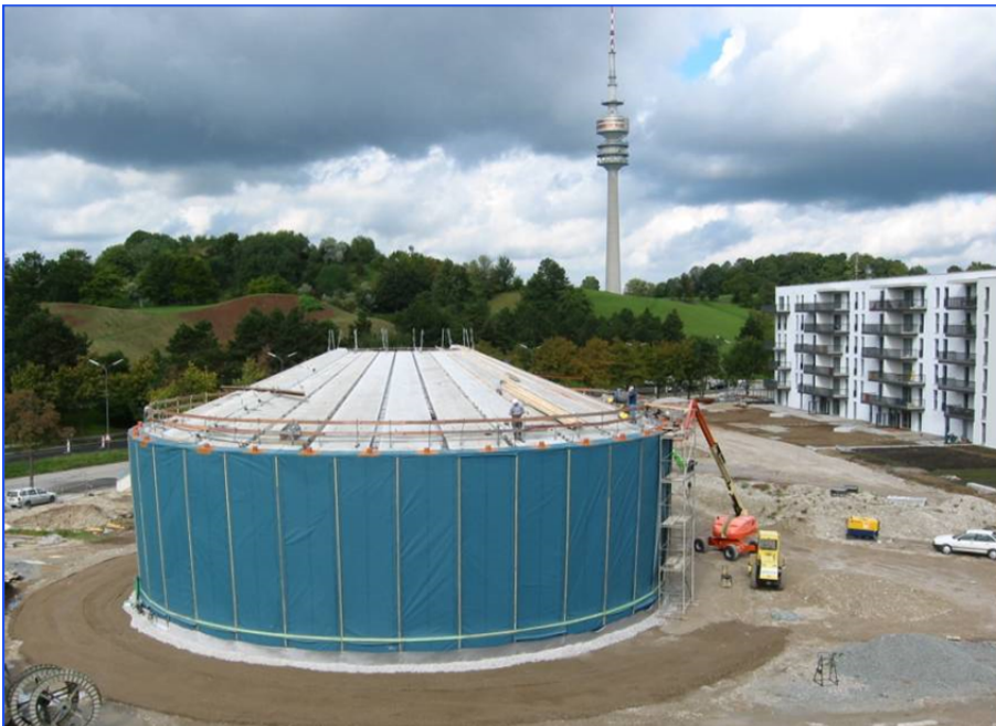
Figure 1. Image of Solar District Heating Network Munich Ackermannbogen – SNAB
