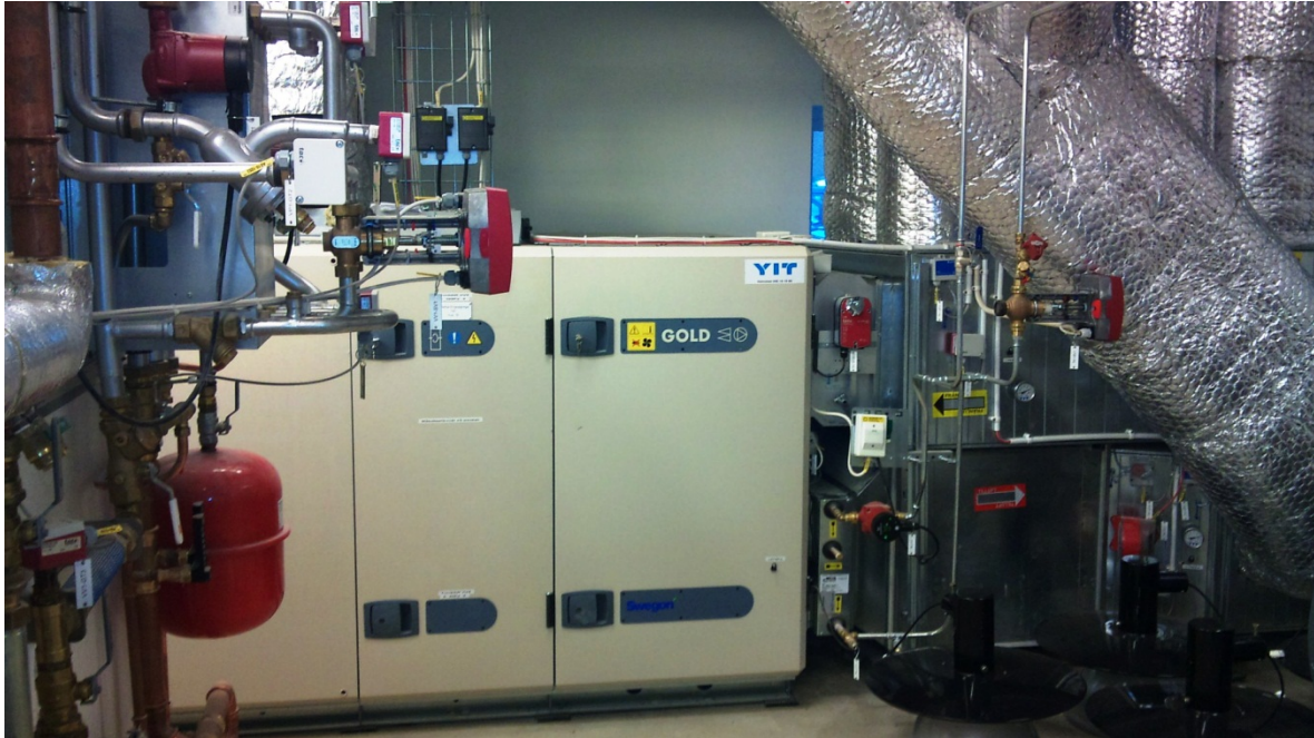
Figure 6. Forced air ventilation system with centrally placed rotating heat exchanger and subsequent district heat added as base load heat supply. Photo: The Author.
