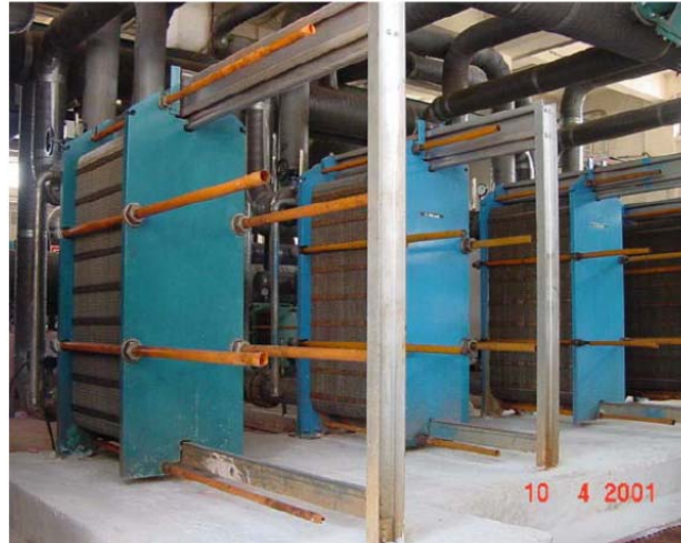
Figure 1 The plate heat exchangers used at Kirsehir DH system [1].
