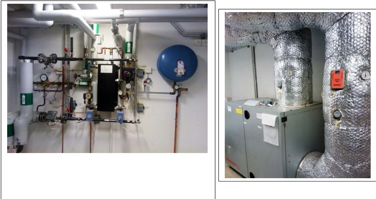
Figure 5. District heat plate heat exchanger sub-station installed at building ground level (left), and installation for exhaust air heat recovery to inlet air (right). Photos: The Author.
