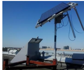
Fig. 2. Fixed unit and two - axis tracking one with the photovoltaic module, solar radiation power density sensor and microinverter
