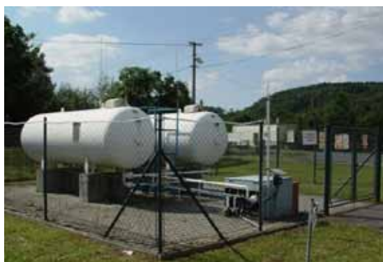
Figure 1 – LPG filling station in a plant.
