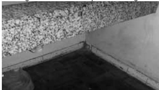
Figure 5 – wall with infiltration and damaged baseboards
