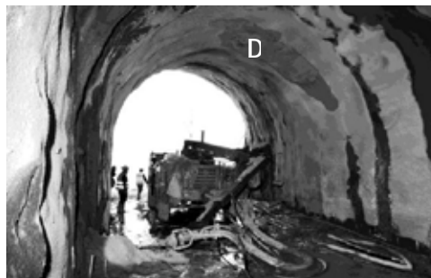
Figure 4 – The area of event: the shotcrete machine and (D, top-right) the area interested by the cementfall.
