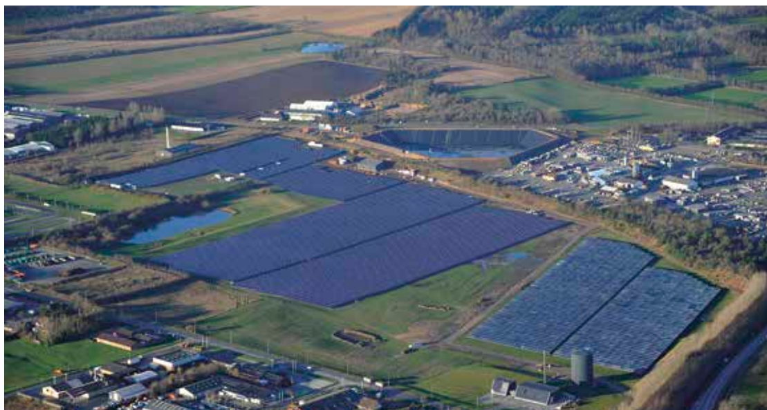
Figure 28 - Vojens solar heating plant with a solar collector area of 70,000 m 2 , the World's largest solar heating system with start of operation in June 2015 [9.8].
