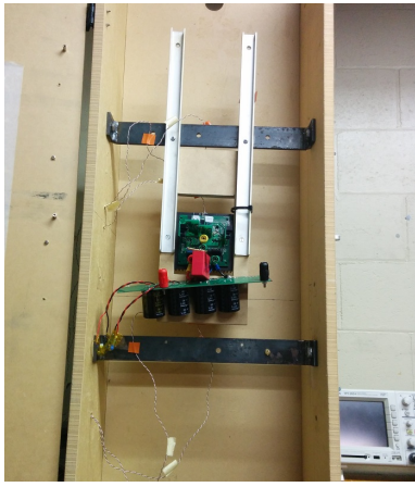
(a) Converter and heat sink in closet
