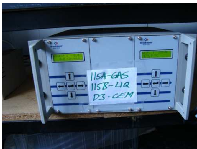
Figure 2.10: Control Box for Flow Controllers and CEM
