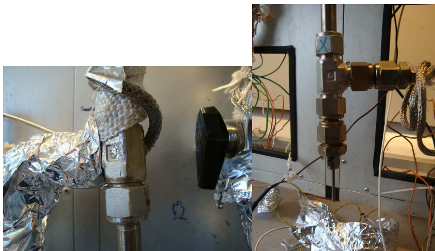
(a) A- Fitting used at the Top of the Reactor (b) B- Fitting used at the Bottom of the Reactor
