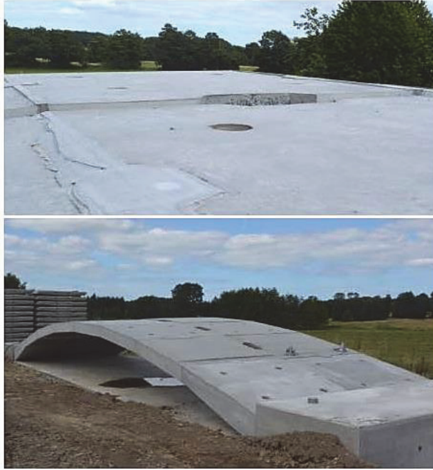
Fig. 8 Top: Close up of difference in height between the two arches at the crown showing the requirement of high accuracy during the assembly process. The first arch (closest) was placed on the foundation three weeks prior to the second arch (furthest away). Bottom: The first 13 m span PC arches in their final position.
