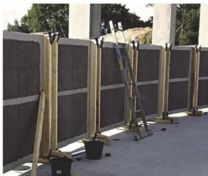
Fig. 7. SL Deck elements on edge positioned on shims on the ground during pour of joints. The bottom of the SL Decks is visible, and the darker areas are the bottom of the light aggregate concrete blocks.
