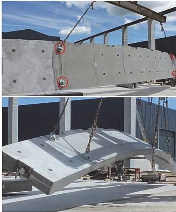
Fig. 4 Top: Lifting points for PC arch (circled in red). The two top points were used for the initial vertical lift. Bottom: Subsequently, the two bottom lifting points were connected, and the arch was rotated, positioned on temporary supports, and transported by truck to the erection site.
