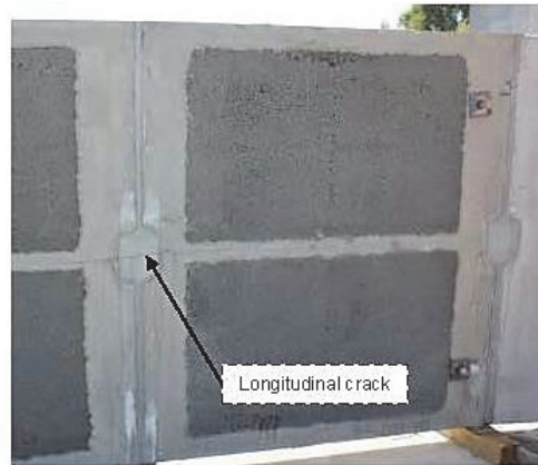
Fig. 7 Crack forming in the longitudinal direction in the bottom of the SL-deck in the joints between SL-elements. Joints between abutment elements and SL-decks did not crack due to larger number of transverse reinforcement. The dark areas are the bottom of the light aggregate concrete blocks.
