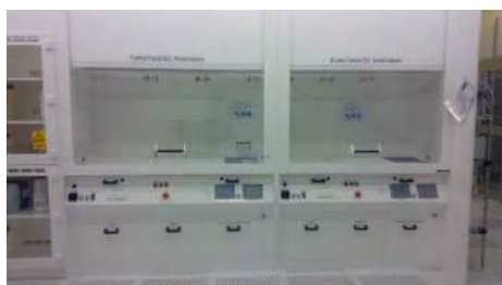
Figure 1: A row of newly installed fume hoods at DTU Danchip. All are equipped with energy saving.
