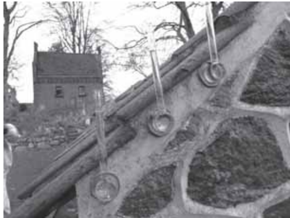
Figure 6. The 25% mortar developed by Ole Jensen was also used by the repair of a wall around the churchyard at Farum church. Picture is taken during measuring of capillarity with the Karsten tubes. (Photo: Martin Jensen)
