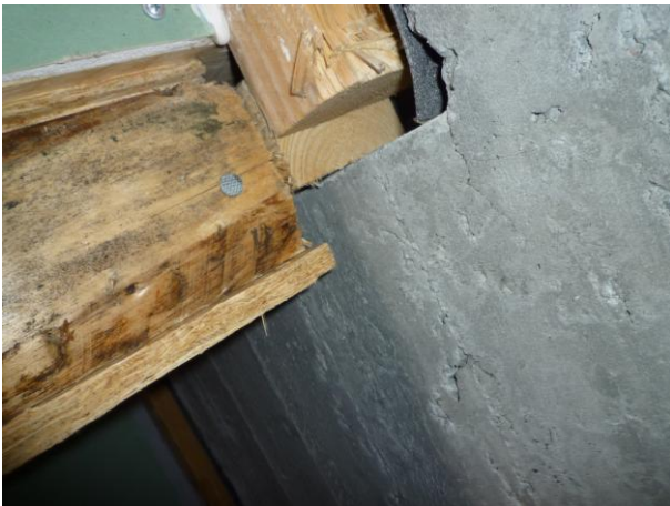
Figure 5: Poor fitting of the materials in a corner to each other. A leaky assembly.
