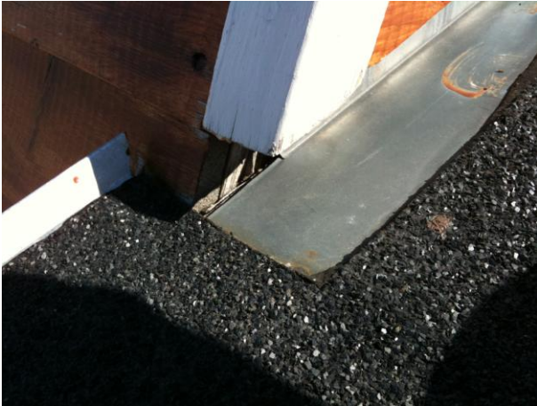
Figure 4: Wrong detailing of a flashing at a roof edge.
