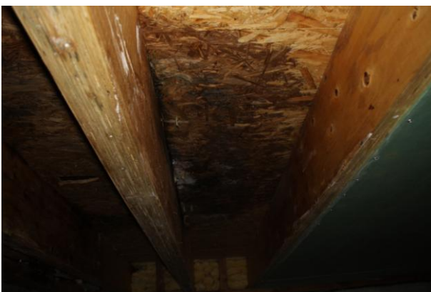
Figure 6: Wetted construction material from leaky construction.
