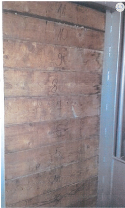
Figure 4. The plank barrier seen from the lashing equipment room. Wood pellets in the cargo hold are visible between planks 10 and 11. The barrier is evidently not gastight. (CORINA). Source: Police photo file #23 [8].
