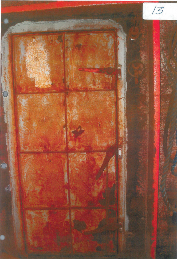
Figure 1. The door in the forepeak compartment, which led the front cargo hold. The door had three closing hinges but only two were engaged. Gasses travelled from the cargo hold to the forepeak through a crevice where the third hinge was not engaged. (AMIRANTE). Source: Police photo file #13 [8].
