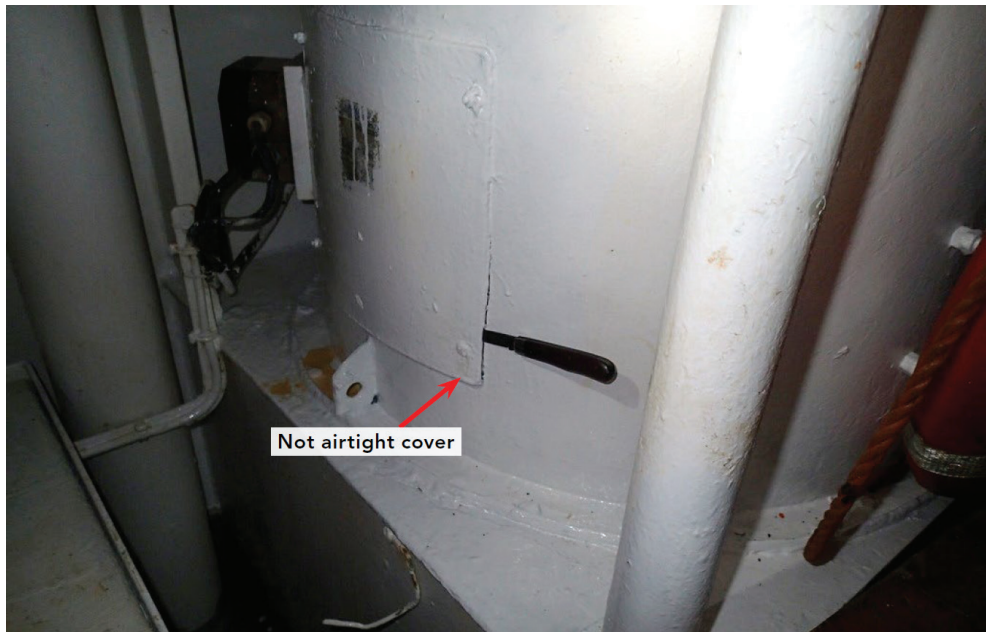
Figure 2. The inspection hatch on a ventilation duct that ran from the cargo hold through the forecastle. A minor gap in a section of the rim (knife blade inserted) allowed gasses to travel from the cargo hold to the bow area. (LADY IRINA). Source: [13].
