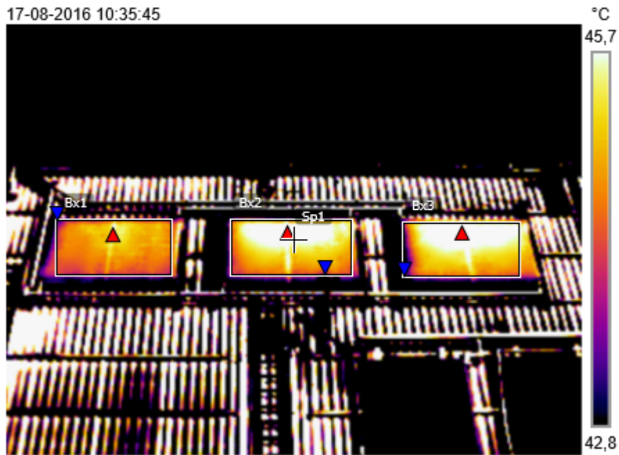
Figure 5: Thermal vision image of PVT collectors during operation in sunny condition.
