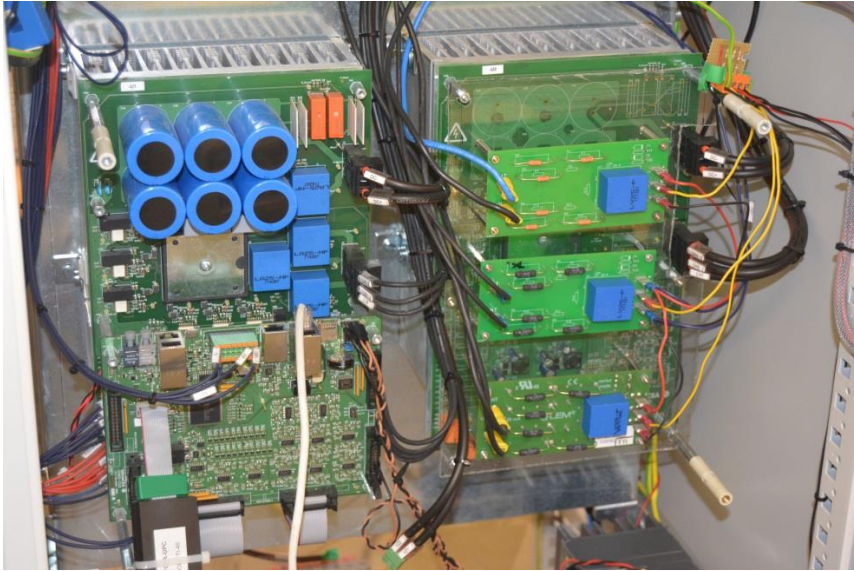
Fig. 5.3 Picture of Measurement and control board inside a converter
