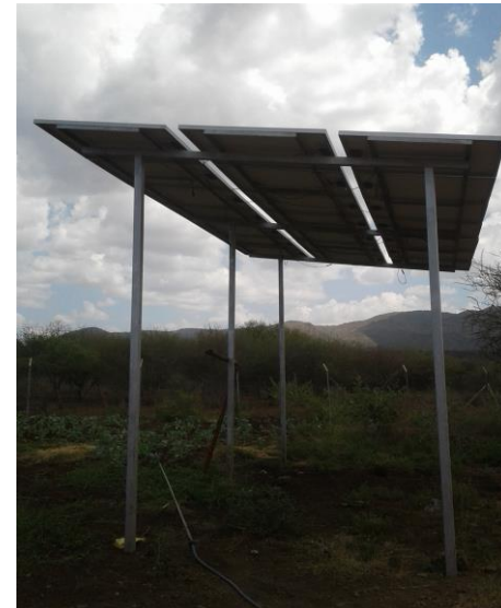
Photo 7: Losambumbur borehole in Baringo supporting small scale farming and livestock use
