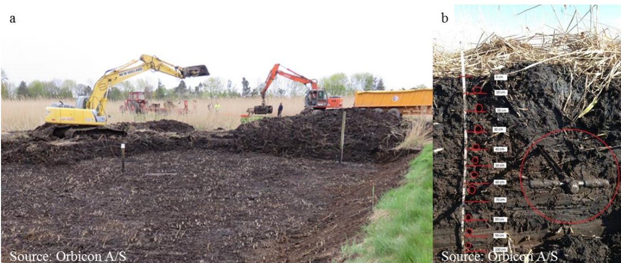
Figure 5. a) Excavation of sludge residue and reeds from a bed in an STRB system. b) As sludge is loaded into the beds over several years, a body of residue builds up. The lowermost layers have resided in the bed the longest. As a rule of thumb, 10 cm of sludge residue corresponds to the build up of one year's supply of sludge.
