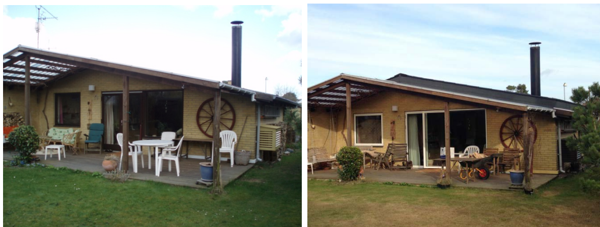
Fig. 9. House A before and after the renovation. Visible changes are the new windows and roof.
