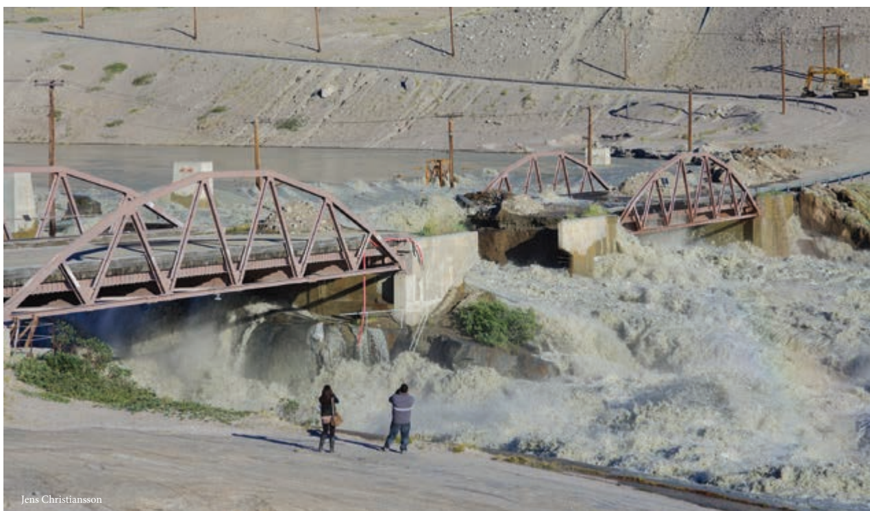
Figure 6.10 Flooding washing out around the Watson river bridge foundations and over the Kangerlussuaq West Greenland water supply pipeline on 11 July 2012.
