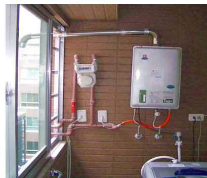
(b). Natural gas water heater
