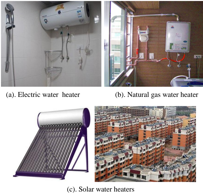
Figure 2. Individual water heater installations in Chinese households
