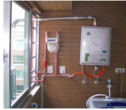
(b). Natural gas water heaters
