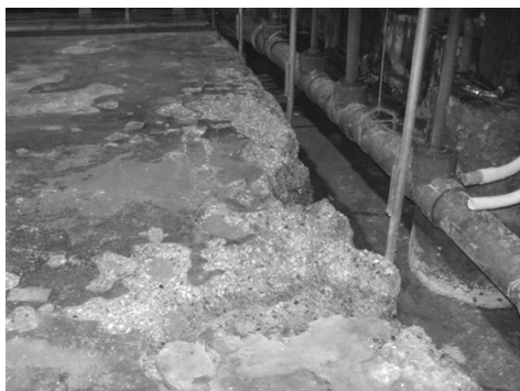
Figure 1.1: Damage on concrete flooring in a chemical etching plant. The floor was exposed to acid drips and spills. Reproduced from [4] with permission from NACE International, Houston, TX. All rights reserved. ©NACE International 2016.
