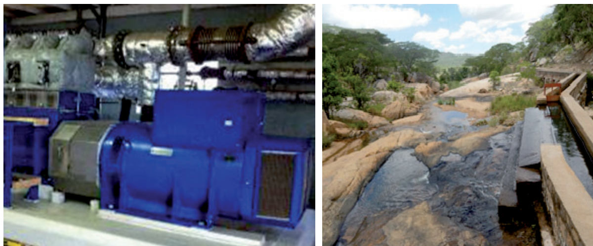
Figure 11.4 Biomass Power plant running on sawmill and wood waste and micro-hydro site
