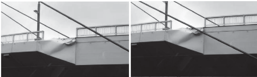
Figure 2.7 – Cable vibrations in dry conditions observed on bridge cables prototype in Japan. From Matsumoto et al., 2010.
