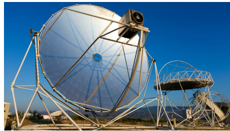
(b) Dish Stirling engine facility [72].
