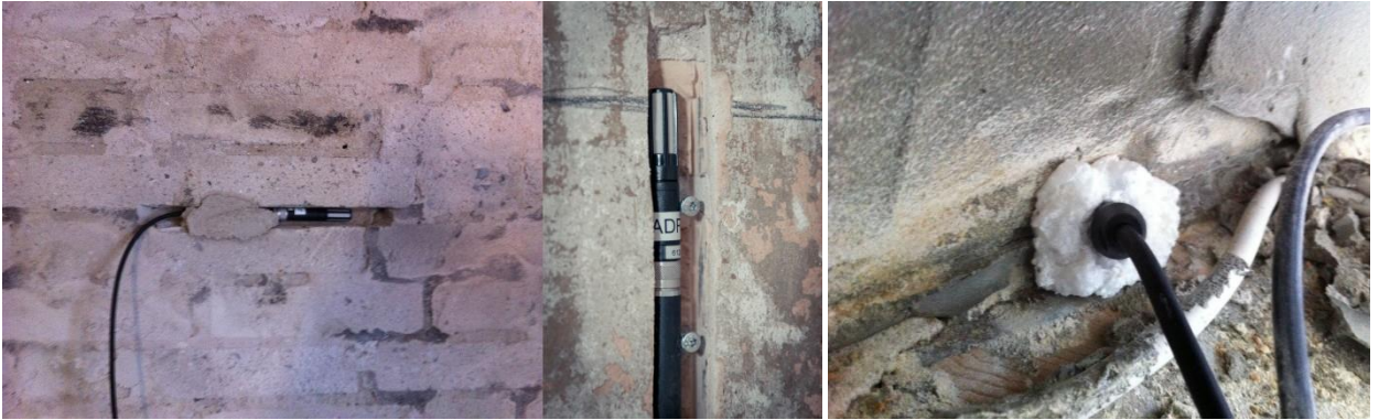
Figure 2: Sensors placed (from left to right) in existing joint, purposely-designed notch, and drilled to beam end.
