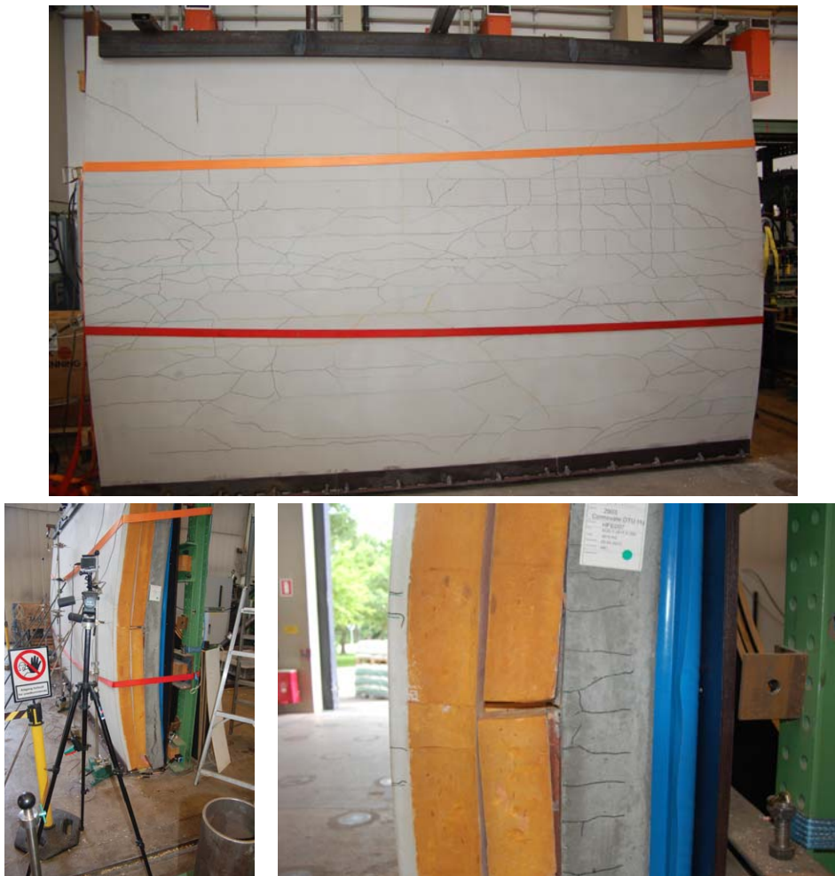
Figure 7.16. Typical failure modes of the panel #01 - test setup 1.
