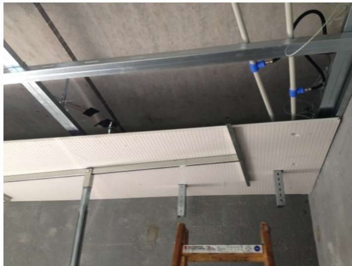
Figure 1: Diffuse ceiling inlet construction and connection of capillary mats to manifold pipes
