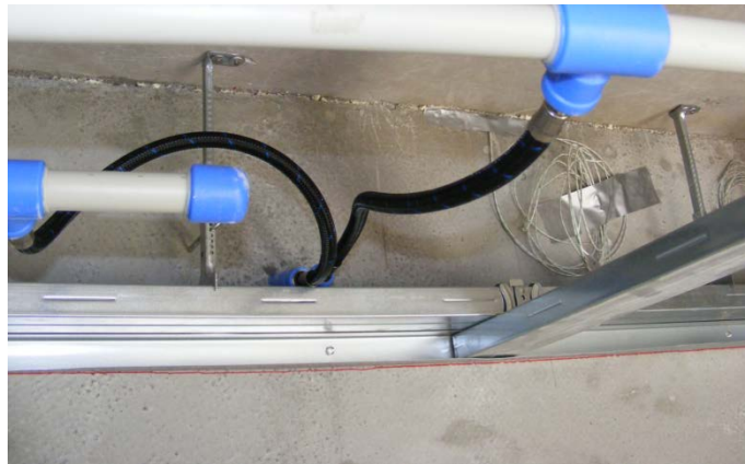
Figure 6: Connections of capillary mats in the wall to the main manifold with flexible pipes
