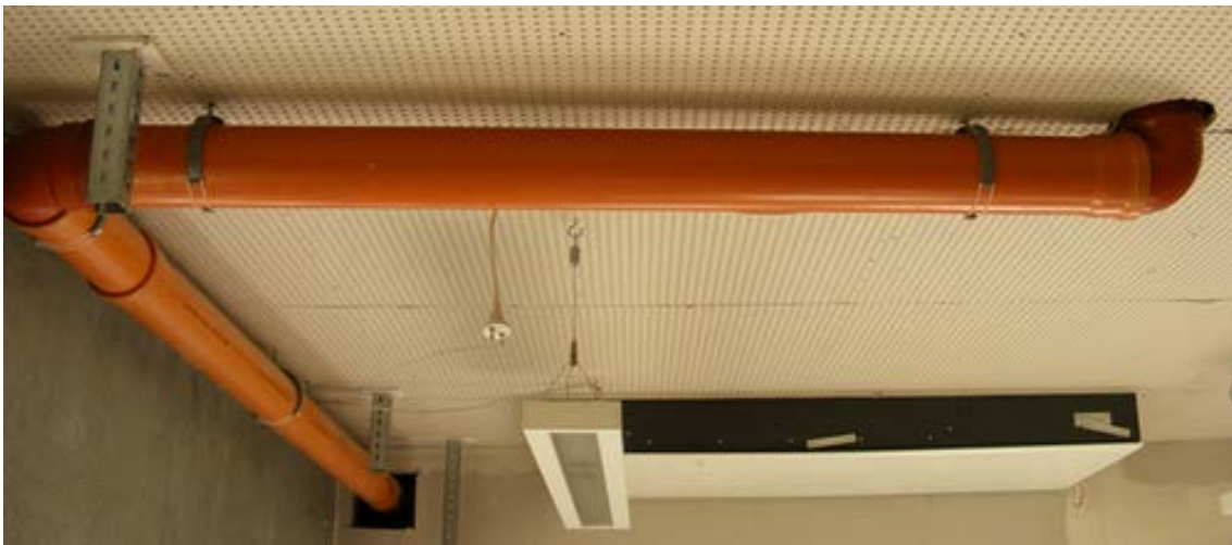
Figure 14: Drainage pipe situated below suspended ceiling
