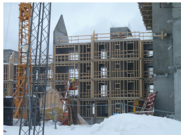
Fig. 2. Example where the traditional building method is used. Gables and interior walls of in-situ cast concrete, façade with timber frame
