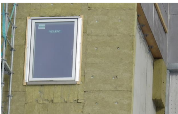
Fig. 4. Building with focus on non-organic materials; outer walls of in-situ cast concrete with mineral wool on the outside. Later a ventilated cladding was installed but no wind barrier.
