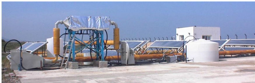
Fig.1.2: Photo of the one-stage pilot plant constructed, including a spray evaporation unit [7].
