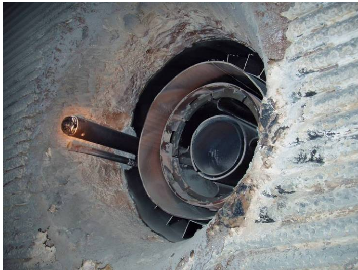
Figure 3 The Mitsui-Babcock Low-NOx burner in dual-fuel configuration.
