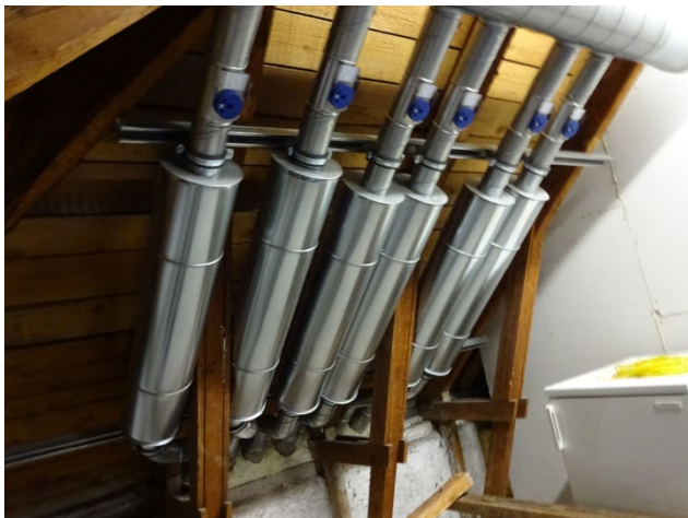
Figure 3-7 Supply air ducts in attic with flow regulation dampers, silencers and penetration to the outside of the exterior wall.
