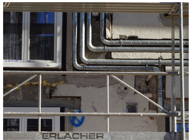
Figure 3-3 View of supply air ducts being routed on exterior wall prior to installing new insulation layer.
