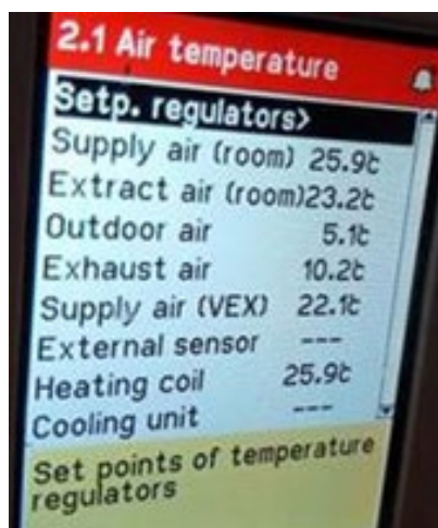
Figure 4-59 Photo of an AHU display that shows temperature measurements in the supply and exhaust.
