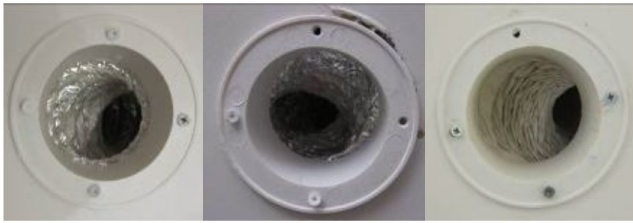
Figure 4-57 Extract terminals with diffusers removed showing constrictions in flexible ducting.
