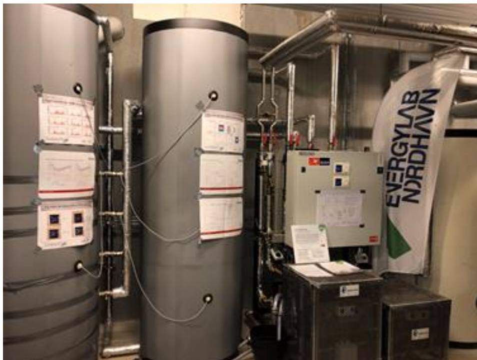
Figure 2: Heat Booster Substation installed and operating in Havnehuset.
