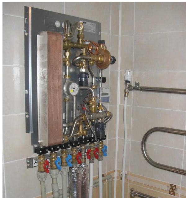
Figure 20. Visualization of individual heat substation and heat meter for every flat
