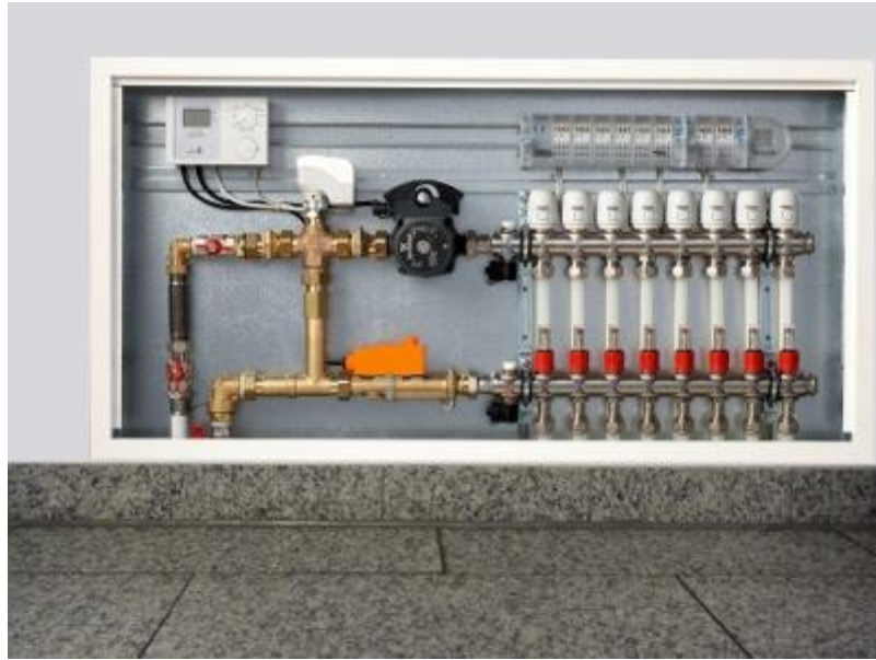
Figure 21. Visualization of heating system collector and individual heat meter for the flat (collector or one floor heating system)
