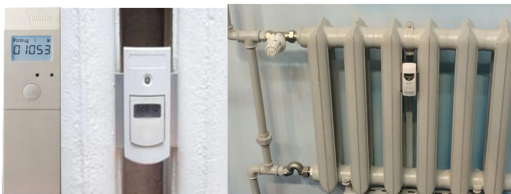
Figure 24. Visualization of metering process by electronic heat cost allocator
