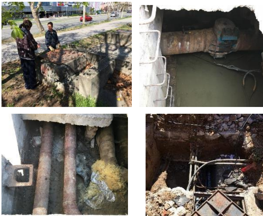
Figure 8. DH network pipes have water leakages and poor thermal insulation
