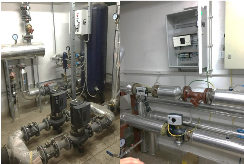
Figure 10. Heat substations in new buildings
