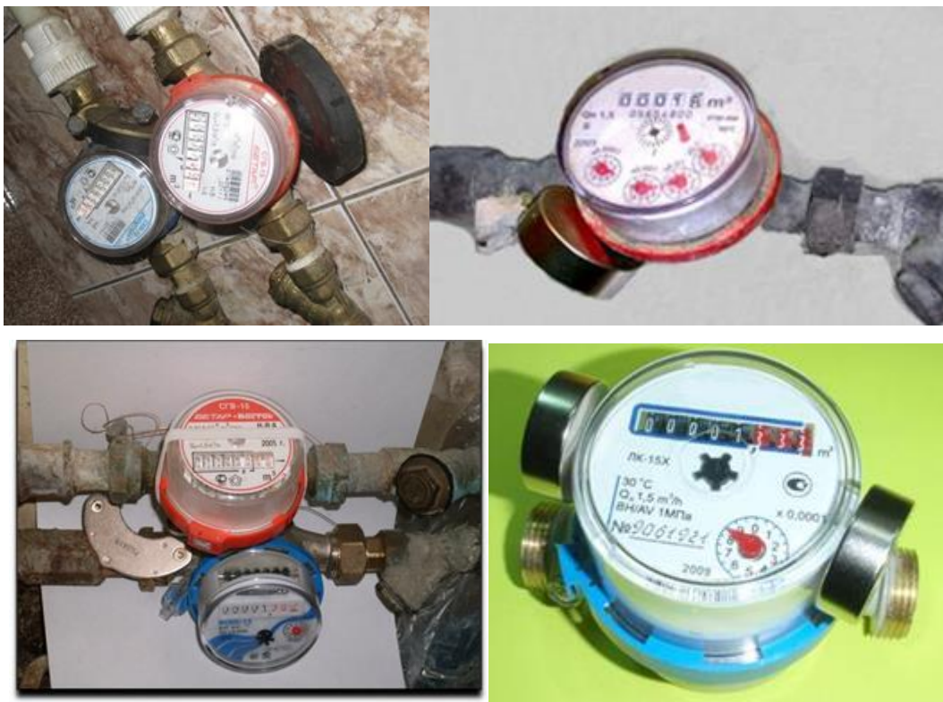
Figure 25. Magnets on water meters
