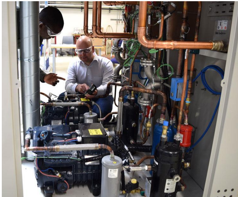
Figure 11: Installed prototype from HeatUp project. Source: [43]
