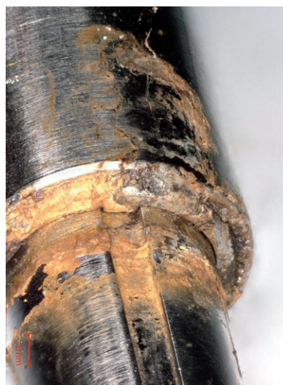
Figure 4. Digital microscopy of the junctional discoloration, i.e., corrosion products.
