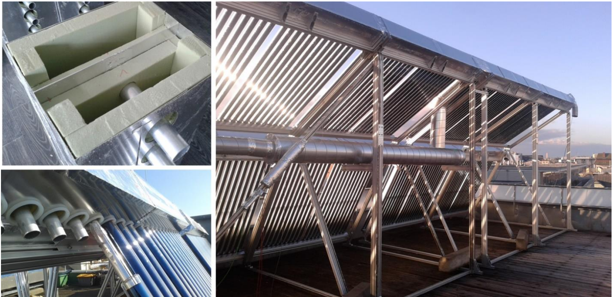
FIGURE 5-45: SOLAR THERMAL HOT AIR INSTALLATION ON TOP OF THE UNIVERSITY-BUILDING (RIGHT), WITH DETAILS OF THE TUBE IN TUBE AIR CHANNEL (LOWER LEFT) AND MANIFOLD CONSTRUCTION (UPPER LEFT).
