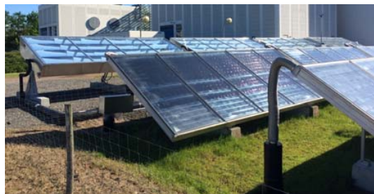
Fig. 3: The CPC solar collector array connecting to flat plate solar collector field in Sæby solar heating plant
