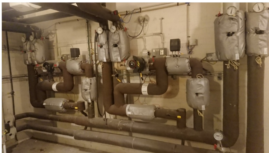
Fig. 2. Substation of the building case.
