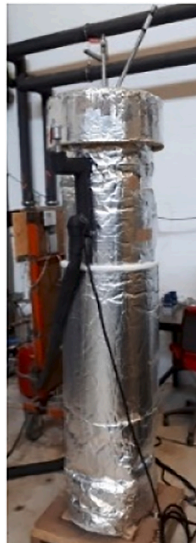
Fig. 1. The investigated heat storage [17].
