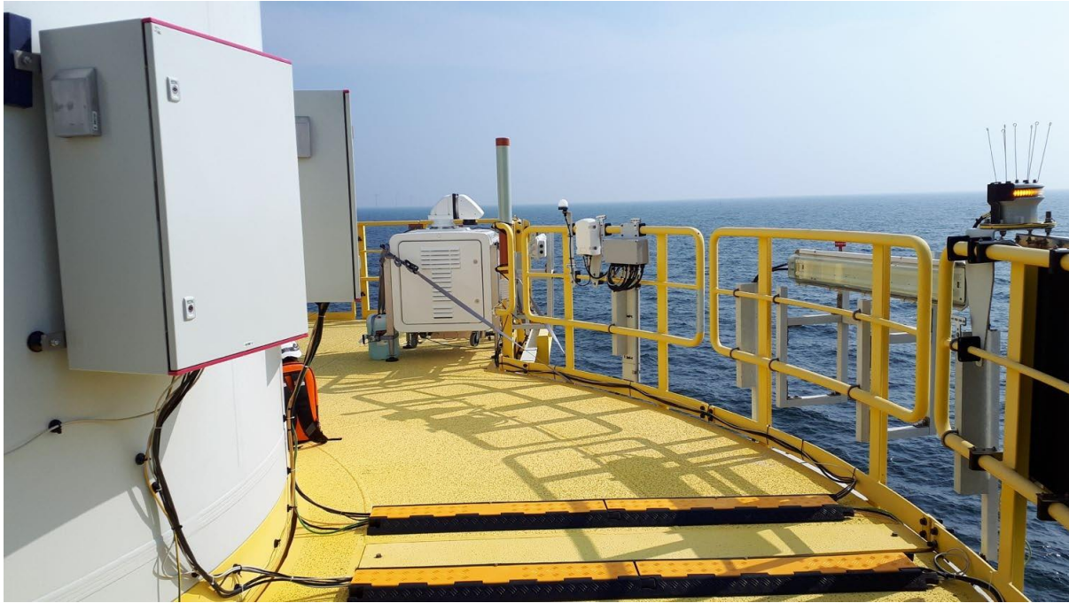
Figure 2 Example of transition piece installed scanning lidar.
