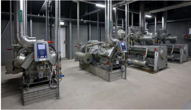
Figure 2: Johnson Controls Heat pumps with UniSAB III controller.
