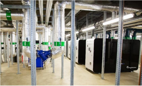
Figure 2: An Energy Machines installation. Heat pumps are located on the right. Sensors are placed inside the boxes.
