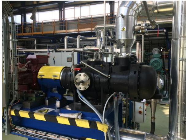
Figure 2-18: SRM prototype compressor skid.
