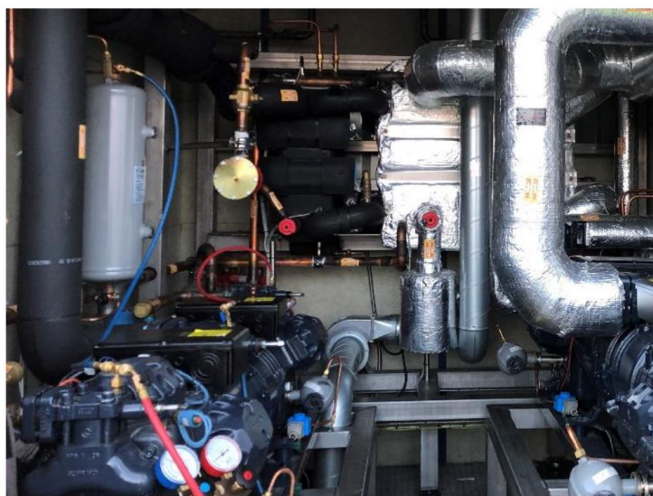
Figure 2-12: Skala Fabrikk - SkaleUP Cascade HTHP.
