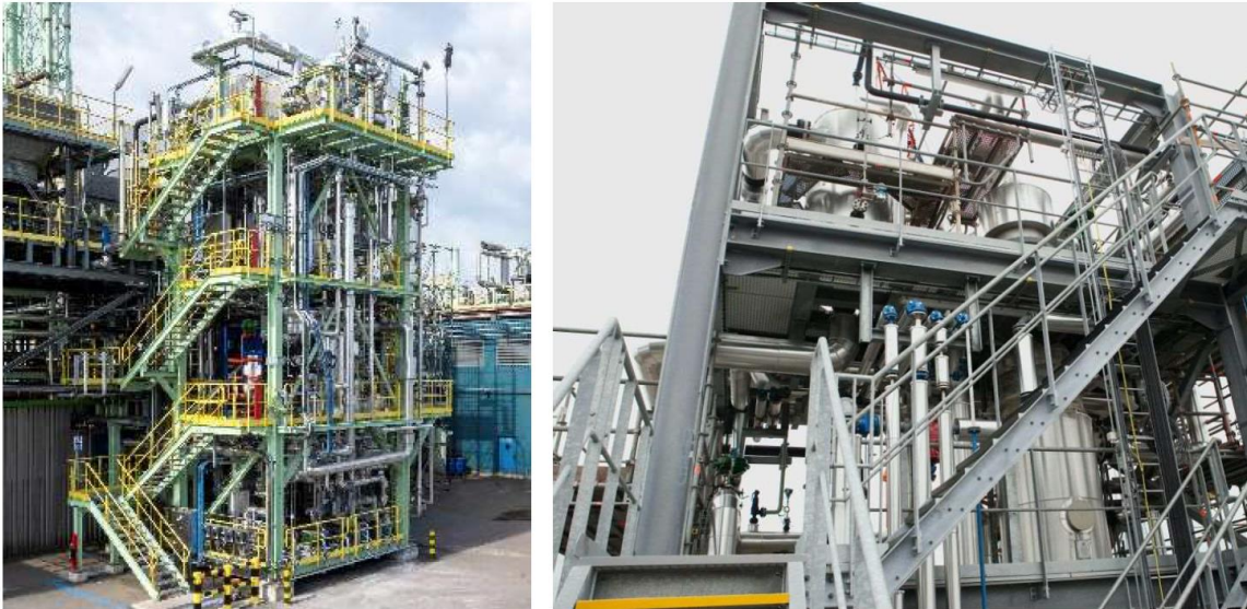
Figure 2-30: Several Pinch Heat Transformer units.
