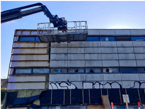
Fig. 5. Manual dismantling of the steel cladding with telescopic handler during the selective demolition process in the case study.
