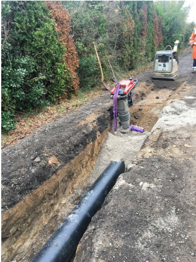
Image 2. District heating pipes for a new housing area in Odense are buried underground on a street that has been closed during the digging work. Photography by the author.
