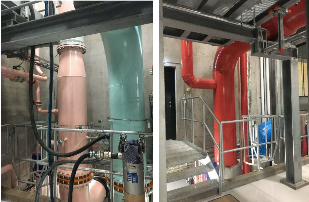
Image 3 and 4. Pipes carrying air and water that connect the district heating heat pumps with the Facebook datacenter. Photographies by the author.
