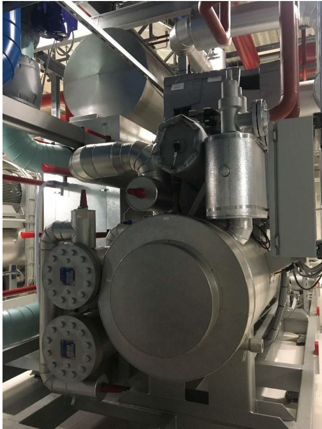
Image 1. One of the new heat pumps built to use server air from Facebook's datacenter for district heating. Photography by the author.
