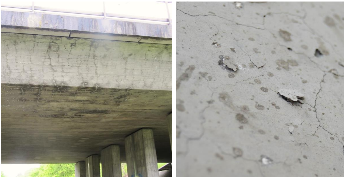
Figure 1: Surface features of ASR damage. Left: map cracking on the deck of an ASR-affected railway bridge on Nivåvej (Nivå, Denmark), courtesy of Ricardo A. Barbosa. Right: pop-outs over porous opaline flint particles (picture size: 5 cm).
