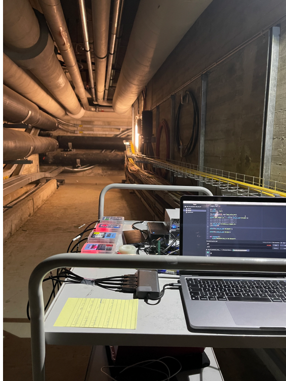
Figure 5.16: Deep indoor environment Hardware Test Setup
