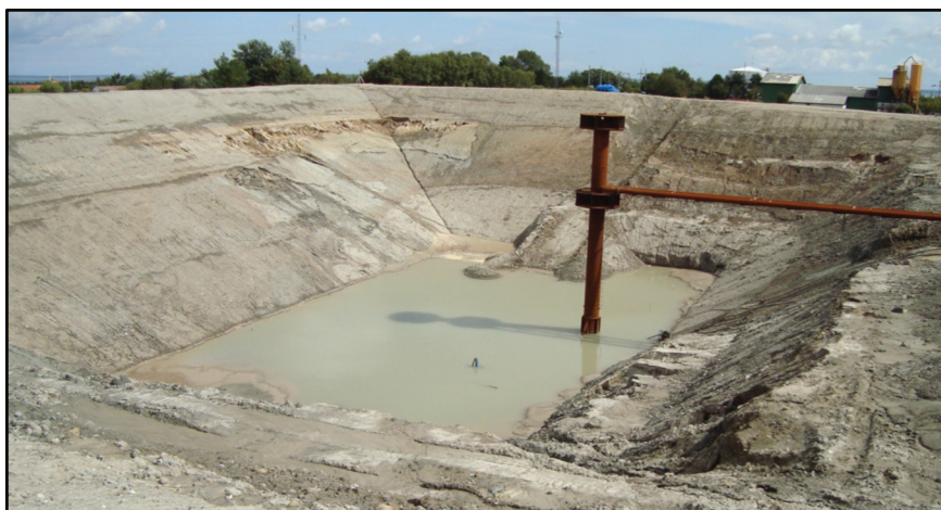
Fig. 2. Diffuser installation in Marstal [22].
