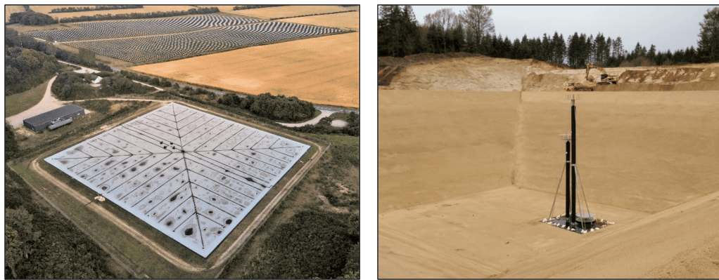
Figure 2.3: Aerial photo from 2015 (left) and diffuser installation (right) from the Dronninglund PTES (PlanEnergi, 2015b).
