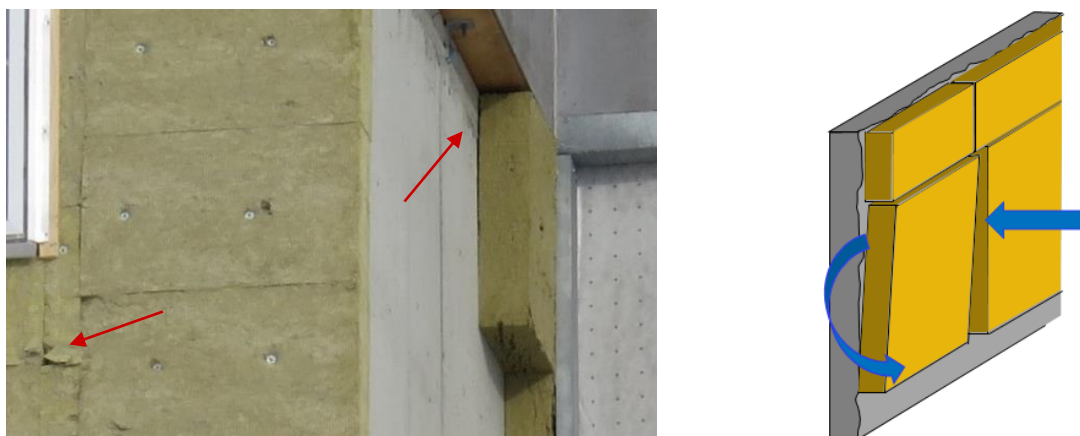
Figure 2. Illustrations of how wind can penetrate the insulation layer due to gaps between insulation mats and uneven concrete surfaces. Left: Photo taken during construction. Right: graphic illustration, which may exaggerate the situation.
