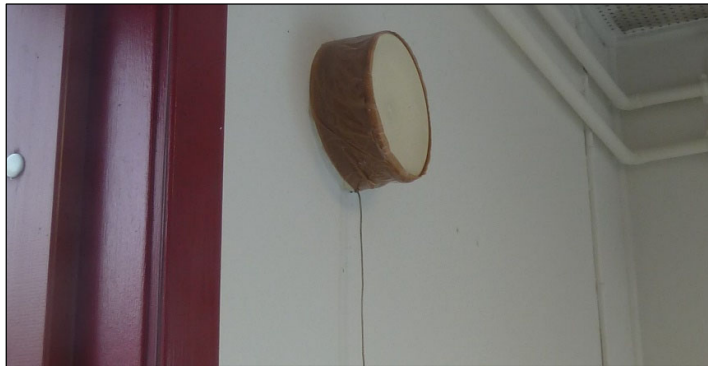
Figure 2.7. Blocked ventilation inlet in Greenland. Credit: Eva B. Møller.
