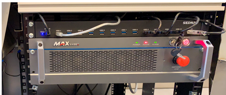
Figure 5.17: Laser from Maxphotonics installed in the system
