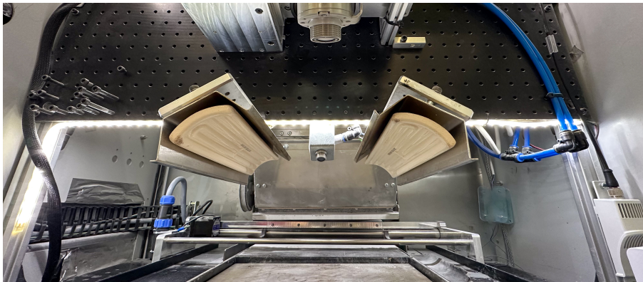
(b) Ceramic heaters installed in the machine
