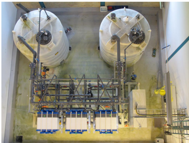
Figure 1.3 Picture of a 15 kW/120 kW·h VRFB system installed as part of the distributed energy systems experimental facility at Risø campus, Technical University of Denmark [40]. The battery stack was refurbished in 2020 and the new stack is 50 kW/120 kW·h.
